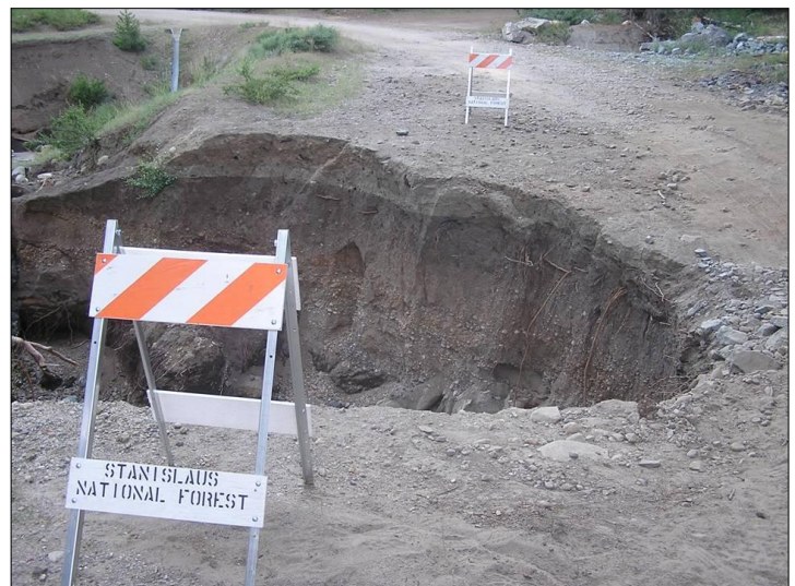
Road washout in the Stanislaus National Forest in California. Unmaintained culverts can lead to road blowouts which results in recreational users losing access to popular destinations. Additionally, many of the agency's roads are unused and unneeded old dirt logging roads. These roads are rarely maintained leading to massive erosion which washes sediment downstream suffocating fish and clogging community water treatment plants. Photo: Central Sierra Environmental Resource Center
