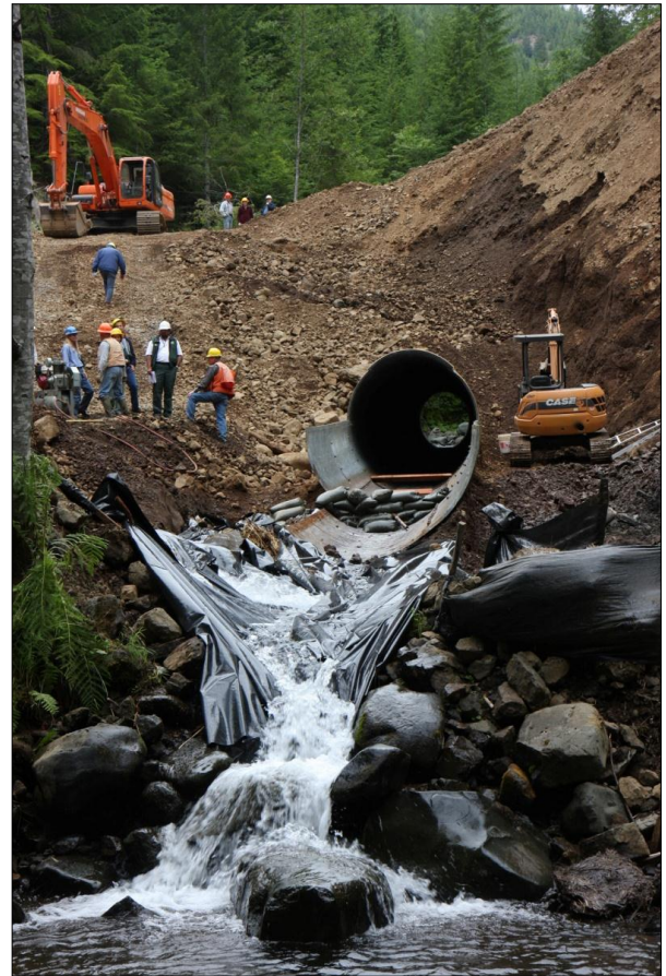
Restoration crew improving water quality and fish habitat on the Olympic National Forest in Washington by removing unneeded Forest Service roads. Road restoration creates high wage jobs for rural Americans. Photo: Steve Zugschwerdt.
